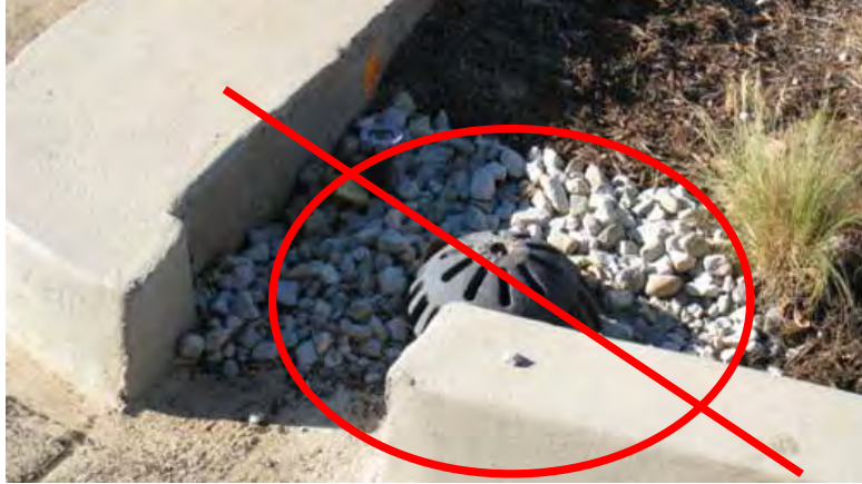
Figure 6: Incorrect Placement of an Overflow Inlet.
