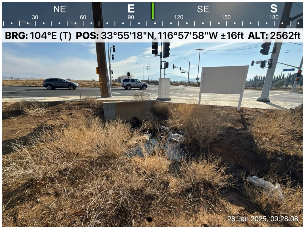
Photograph 4: Drainage culvert at corner of 1 st Street and Pennsylvania Avenue on north side of 1 st Street.
