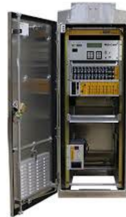
Figure 3-2: Example of 352i ATC Cabinet
