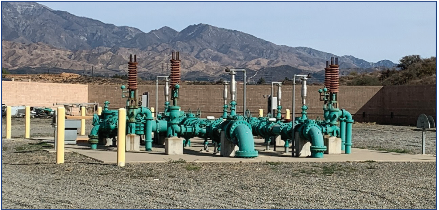
Above Grade Piping at Beaumont Mesa LS
