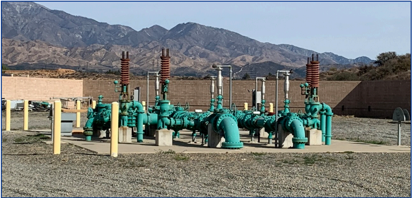
Above grade piping to be replaced at Beaumont Mesa Lift Station
