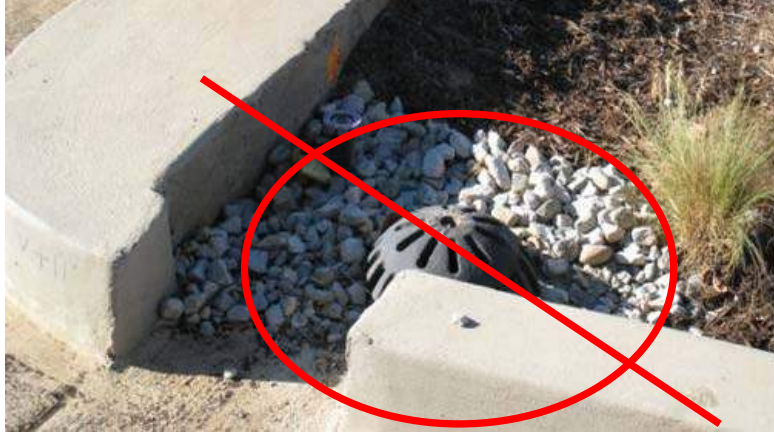
Figure 6: Incorrect Placement of an Overflow Inlet.
