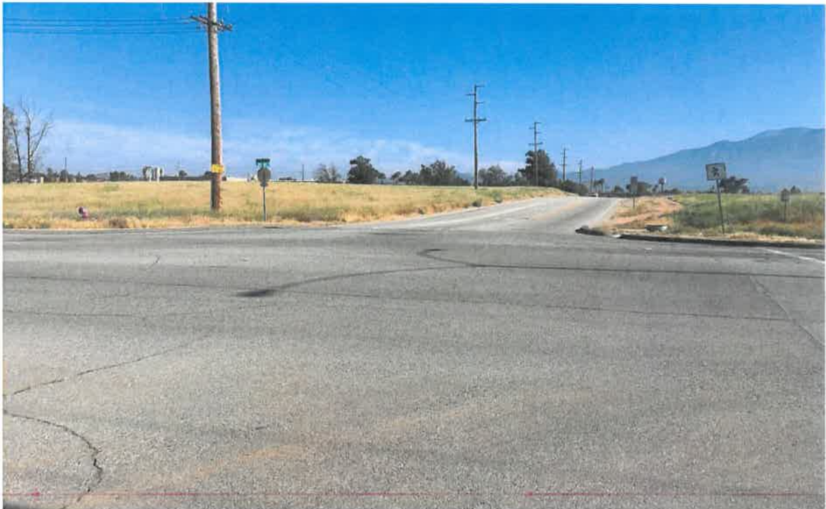
Photo No. 5: This photo shows the conditions of Pennsylvania Ave. from 1 st Street facing north.
