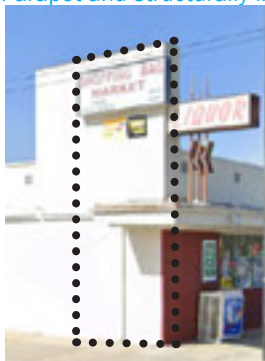
Example of parapet extension on historic building in Beaumont with bounding box for blade sign conformance.
