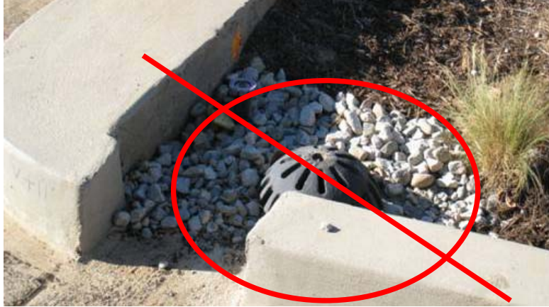
Figure 6: Incorrect Placement of an Overflow Inlet.
