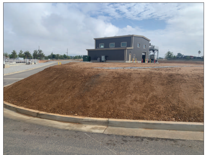
Photo 3 - Graded slopes need protection from erosion
