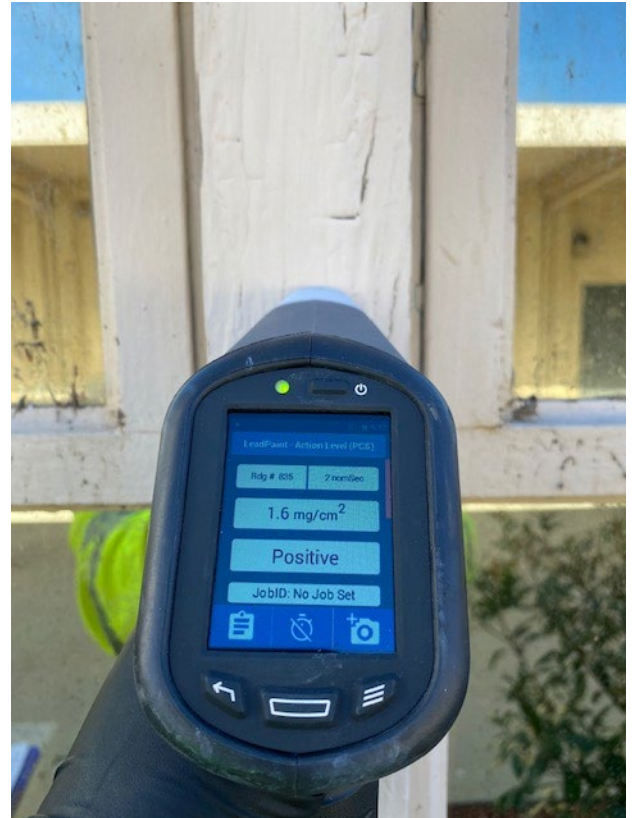
Picture 2: Lead-based paint was detected on the exterior window and window frame of Building B
