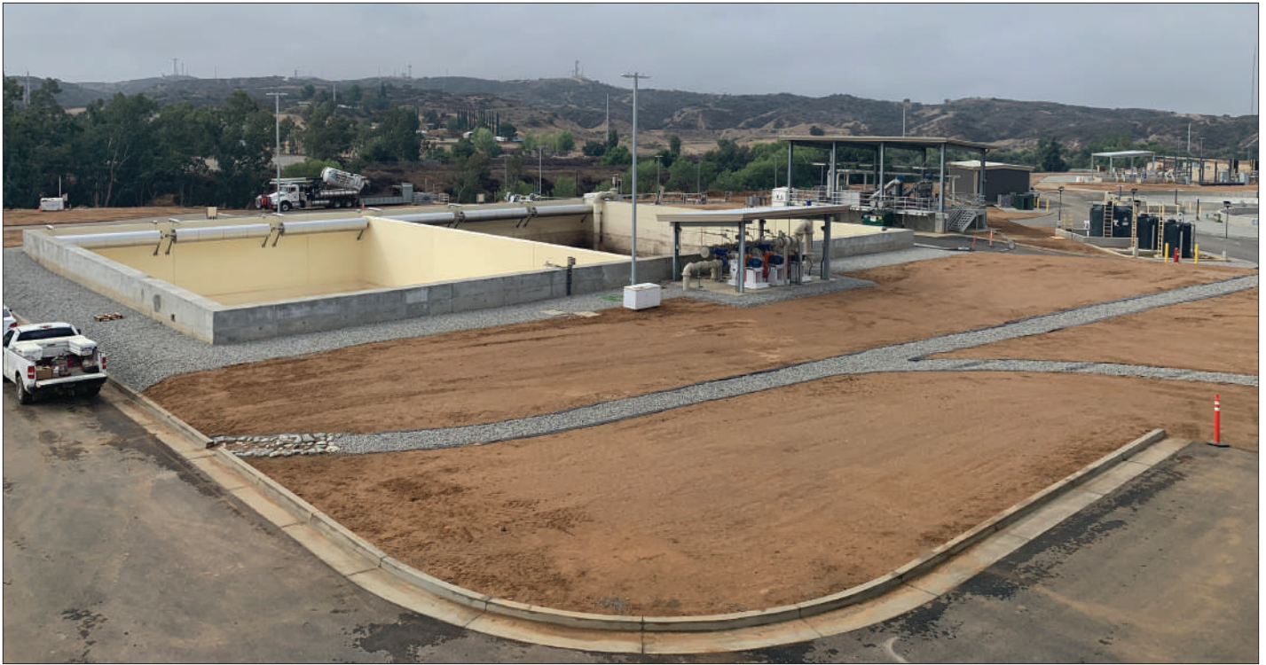
Photo 4 - Area between the Sludge Building and EQ Basin will be paved to create 10-15 new parking spaces for the operations team to utilize.
