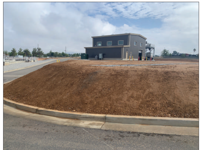
Photo 3 - Graded slopes need protection from erosion
