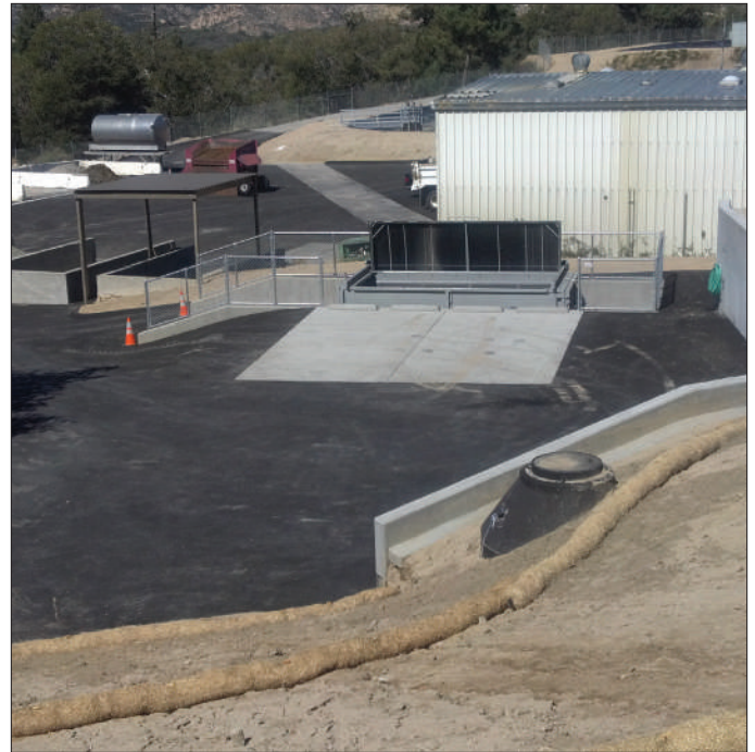
Photo 6 - Willow Creek Vector Station, Lake Arrowhead Community Services District - Showing a roll-off dumpster with an integrated screen to remove solids from the liquid prior to discharging the liquid into the influent sewer.
