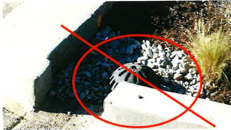
Figure 6: Incorrect Placement of an Overflow Inlet.
